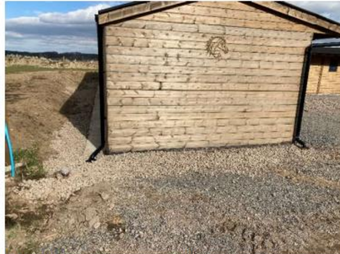
IMG_004 Surface water drainage around outside of stable complete.
